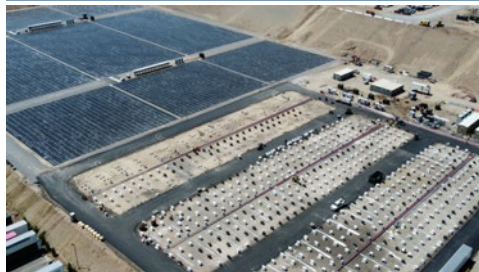
Redwood BESS + Erthos PV Microgrid
