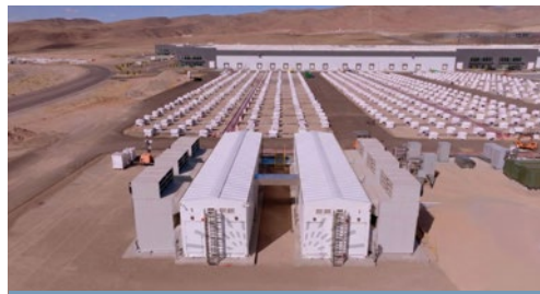
Crusoe-owned modular AI manufacturing facility
